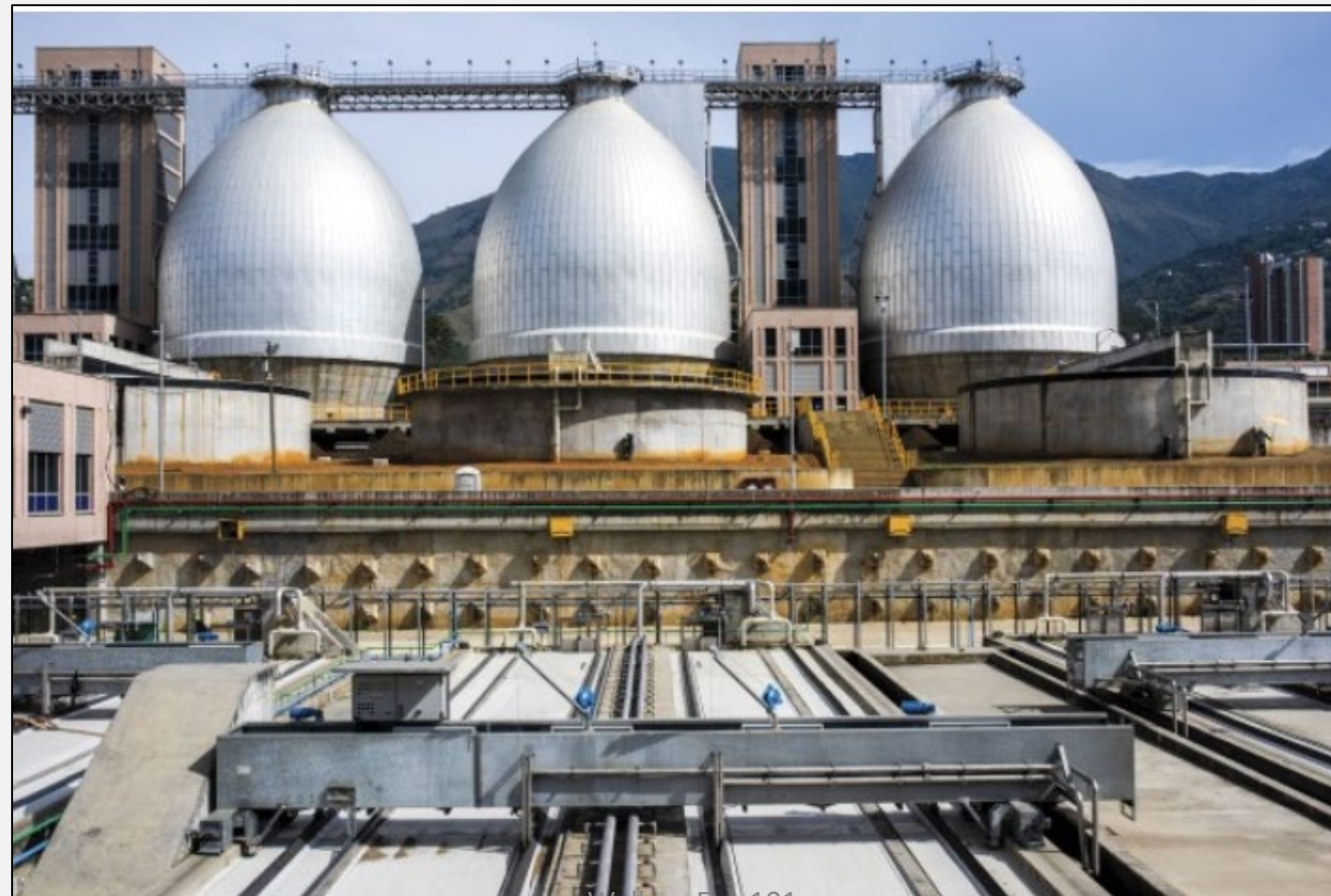
Wellmer Env 101 Medellin's new treatment plant helps reuse wastewater and produces biogas.
